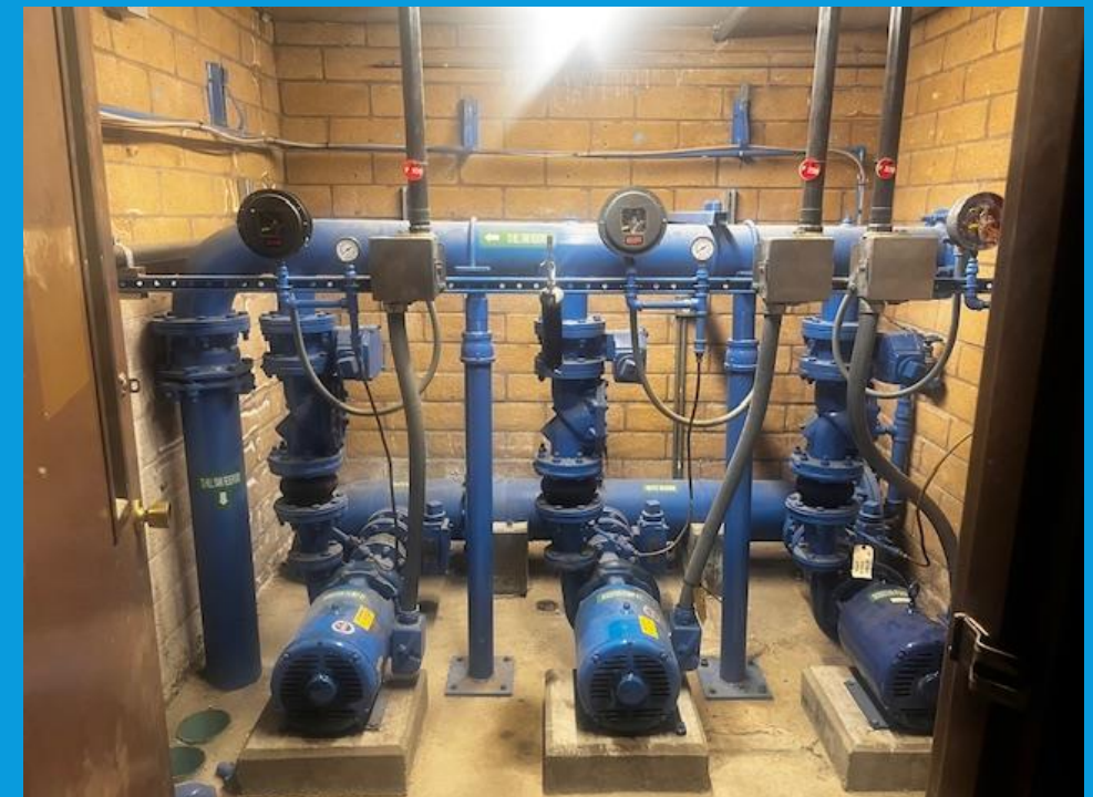
PS from Office Tank to Hill Tank (located at WTP)
