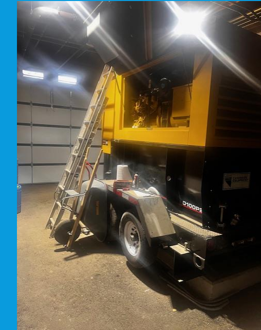
A standby generator for power outages
